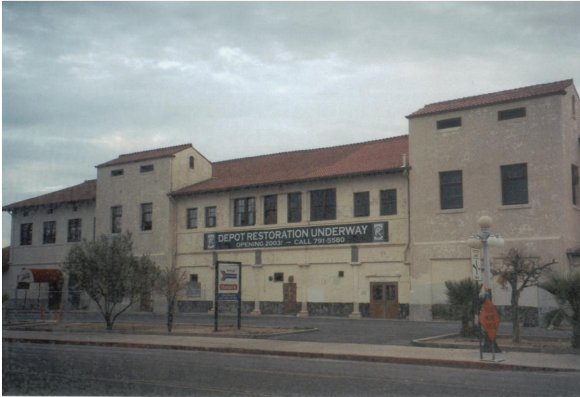
Figure 32. Downtown Tucson Train Depot Undergoing Restoration For Inclusion In The Downtown Tucson Intermodal Center
